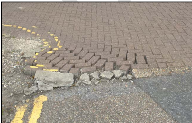
Footway trip, slab profile/rocking slab (SLPF)
